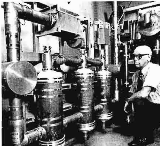
Chief Engineer Don Ferguson shown with filterplexer for TT-35FH. The Ch. 10 transmitter is manned only part-time for handling routine maintenance.
