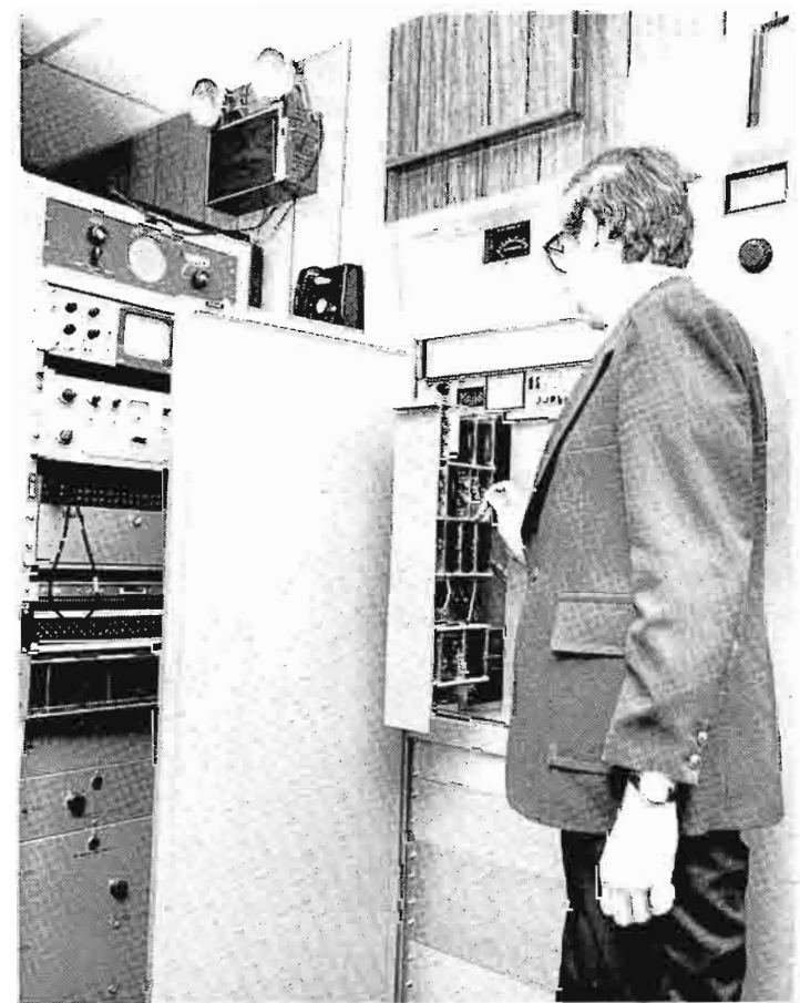
Chief Engineer Larry Vehorn checks TTUE-4A solid state exciter added to upgrade the station's transmission facilities.
